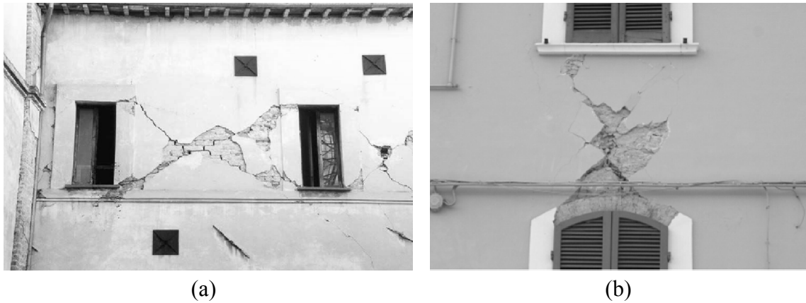
Figure 1.9 – Example of shear failure of: (a) piers (Penna 2008); (b) spandrels (Dazio and Beyer 2010).
