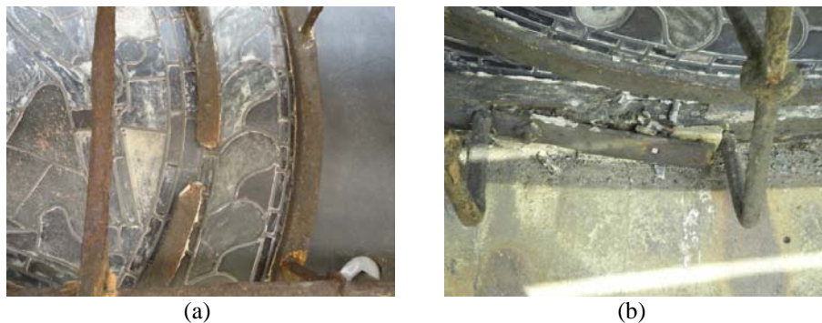
Fig. 5 Visual inspection of the Ferramenta: (a) Broken section; (b) Old repair
