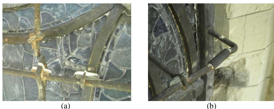
Fig. 6 Visual inspection of the Grille: (a) Broken section; (b) Old repair
