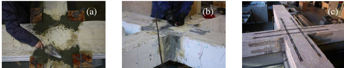
Figure 4. Specimens repair and strengthening: (a) joint reconstruction; (b) crack sealing; (c) MDL-CFRP application.
