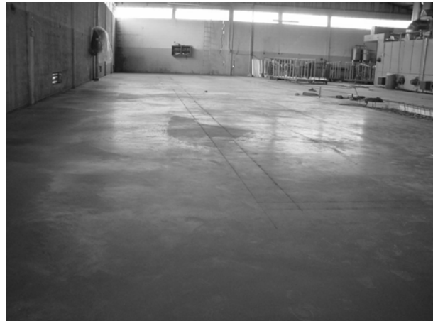
Figure 19 – View of the concrete slab after has been strengthened using a SFRC over-layer.
