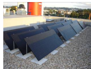
Figure 6. Hot water solar collectors (thermodynamic system).
