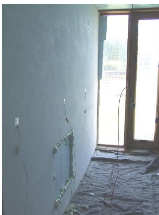
Figure 5.7.2. West room of the adiabatic test cell – Gypsum-PCM façade.
