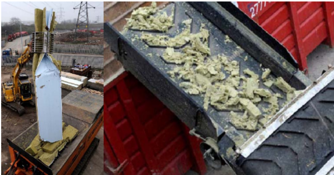
Figure 3.6. Composite panel recycling machine and separation of mineral wool from steel fraction (BRE, 2008).
